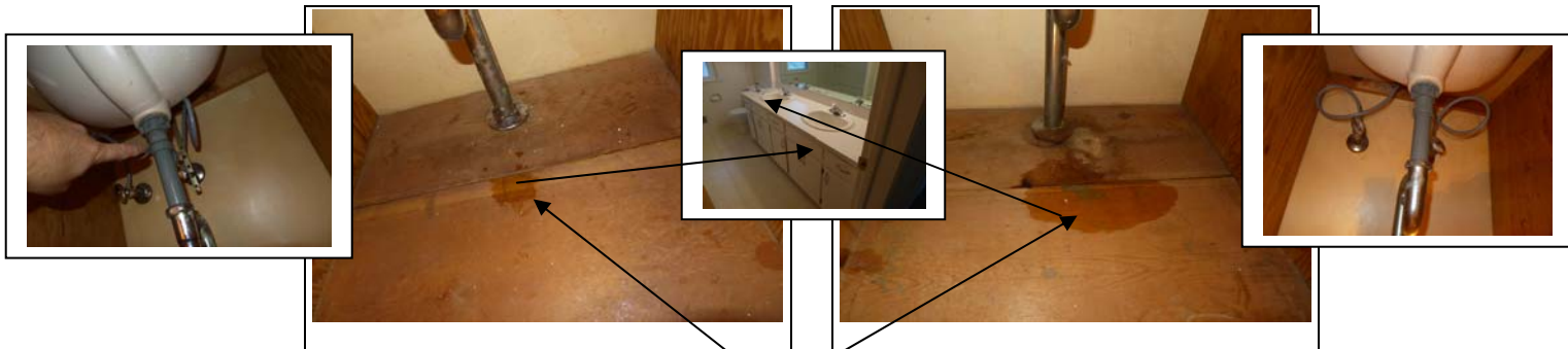
1 st Floor Bath Sink Drains Leaking
