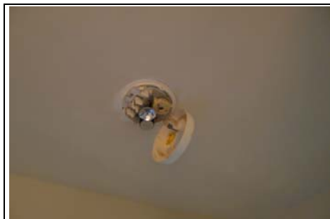
Smoke & Carbon Monoxide Detector Improvements
