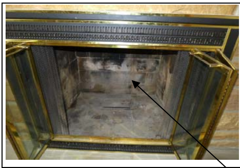
Clean/Inspect/Repair FP Damper (seized/rusted) & Chimney Flue before Settlement/Use
