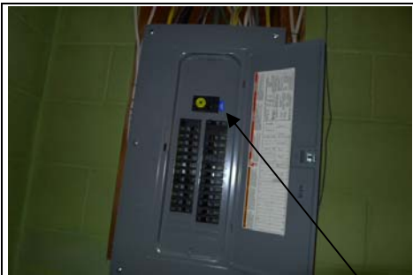
Newer - 100 Amp Main Breaker Panel
