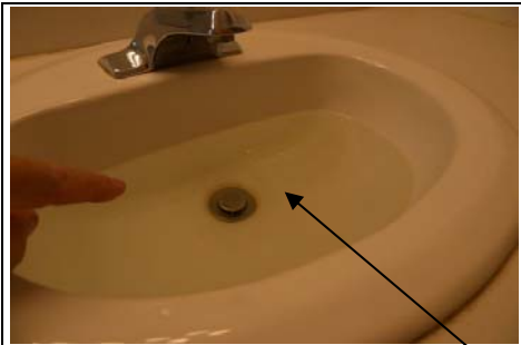
1 st Floor Bath Sink Drains Slow (obstruction?) – Venting Suspect
