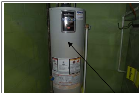
Newer 40 Gallon Gas Water Heater
