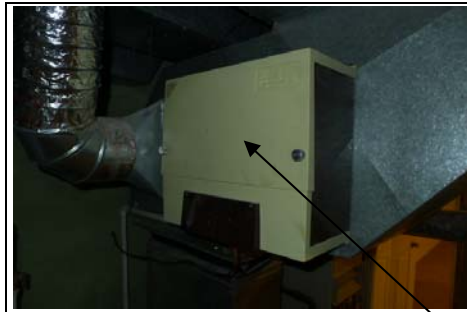
Humidifier – Annual Service Recommended
