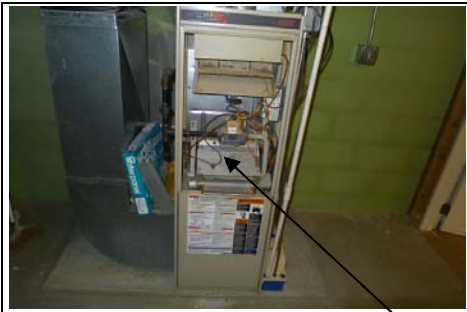
20+ Yr Old Gas Forced Air Furnace – Recommend Annual Service Contract
