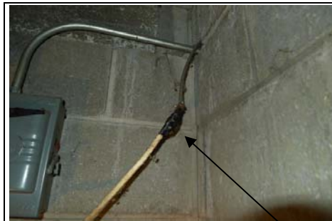
Open Splice – Old Well Pump
