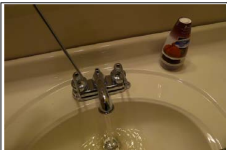
Secure Loose Basement Bath Sink Stopper
