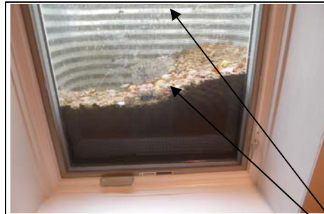
Safety Hazard – Remove Debris from Egress Window and Install Ladder
