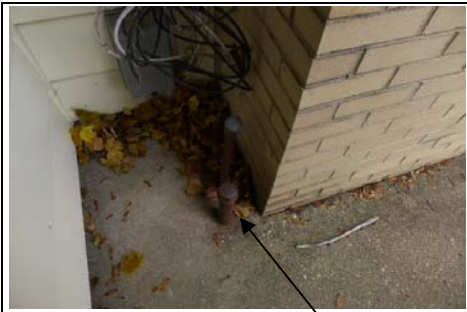
Possible Buried Oil Tank
