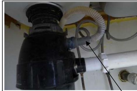
Secure Loose DW Drain Line @ Disposal Disposal Excessively Noisy
