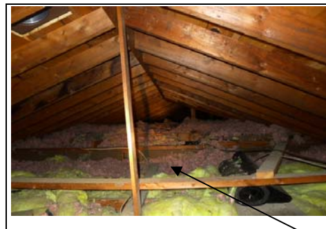
Recommend 18-20” Attic Insulation (total)
