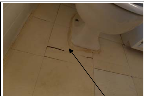
Prior Damage – Toilet Leak
