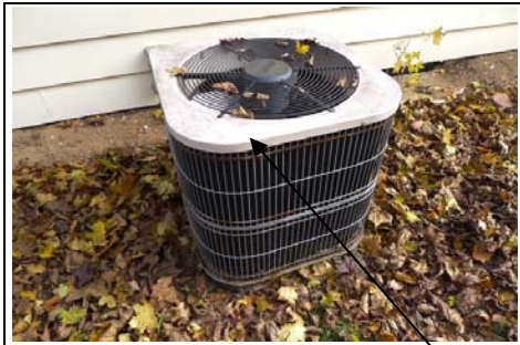
20+ Yr Old AC Condenser – BFR Recommend Service before Settlement
