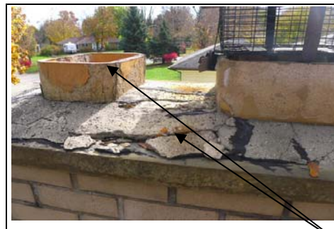
Repair Masonry Chimney Cap – Spalling Recommend Weather/Pest Cap
