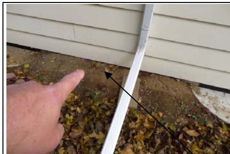
Insufficient Clearance between Ground & Siding
