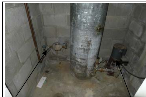
Water Meter/Main Shut-Off Valve Old 2" Shallow Water Well
