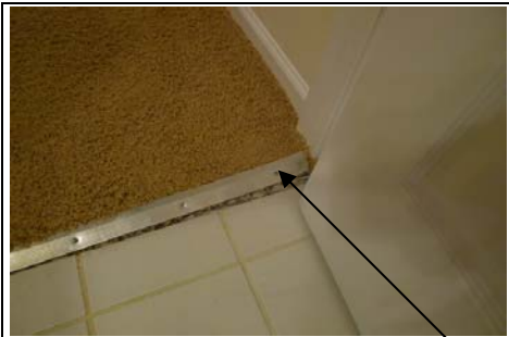
Basement Bath Floor Trim Loose (Trip Hazard)
