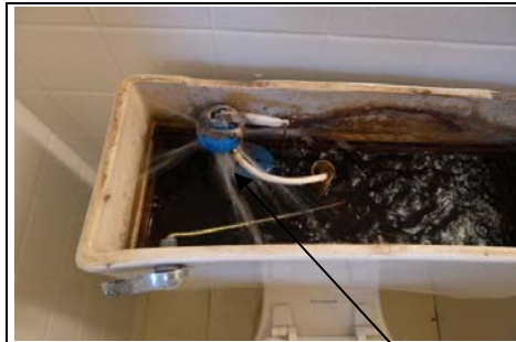
Repair/Replace Toilet - Leaking
